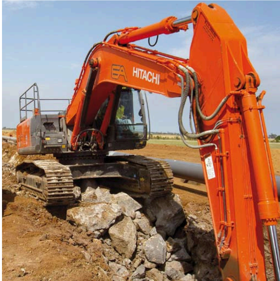
FuelGuard has stopped fuel theft from EA Hire's equipment at the Brooklyn-Lara gas pipeline project.
